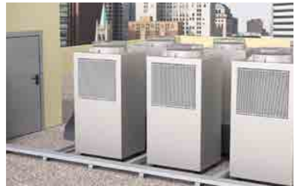
Rooftop HVAC Installations
