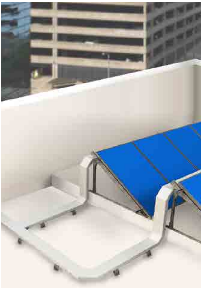
Rooftop Solar Installations
